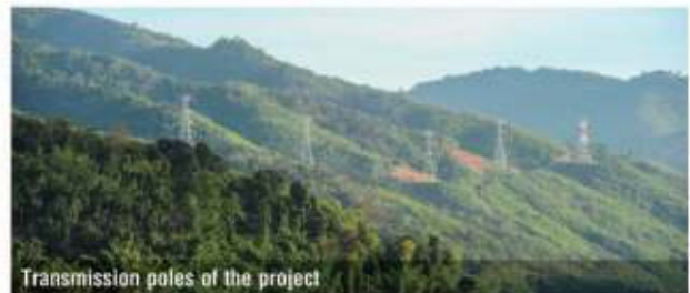
Transmission poles of the project
