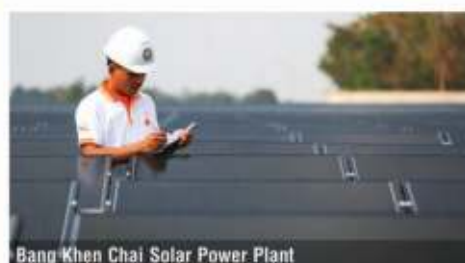
Bang Khen Chai Solar Power Plant
